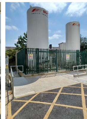
VIE Oxygen Plant - creation and installation of two new oxygen tanks and supplies to main ITU wards in C block.
