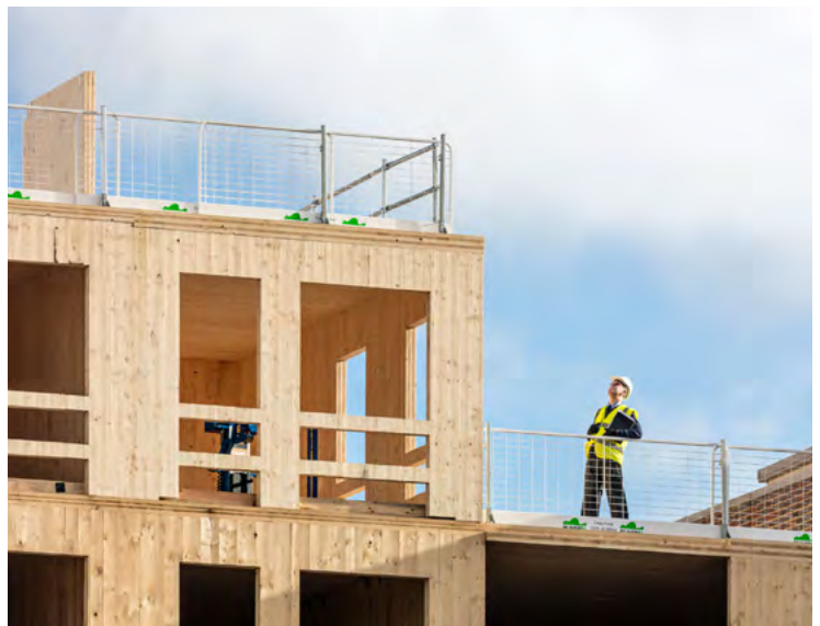
Fig.8.7 - This ground-breaking use of cross-laminated timber technology significantly reduced the carbon footprint of the building in terms of the amount of material used and energy consumption. (Dalston Works by Waugh Thistleton Architects ) [Credit: Waugh Thistleton Architects]
