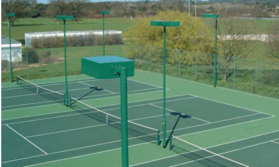
HI-LUX – Match107/WB 17B fittings installed on tennis courts with the type of columns proposed for Canons Leisure Centre
