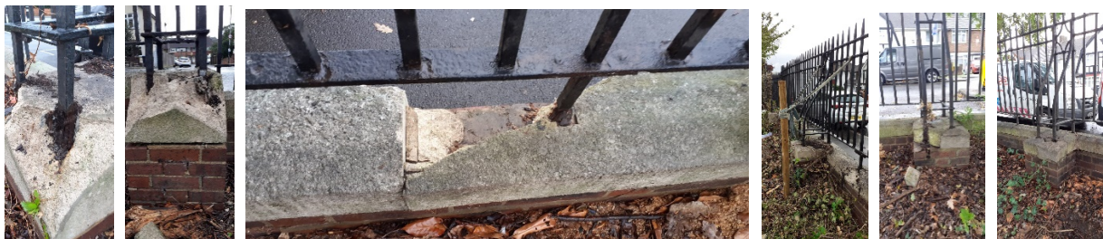
MSJC Garth Road railings integrated into the existing brick piers and perimeter wall line
